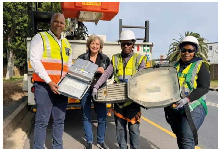
Light-bulb moment: From left are Cllr Siseko Mbandezi (acting Mayco member for Energy) and Ald Theresa Uys (Mayco member for Corporate Services), holding one of the new, energy-efficient LED streetlight fittings that have been installed in Durbanville to replace the older, dimmer and more power-hungry bulbs, like the one shown by the two City Energy officials.
